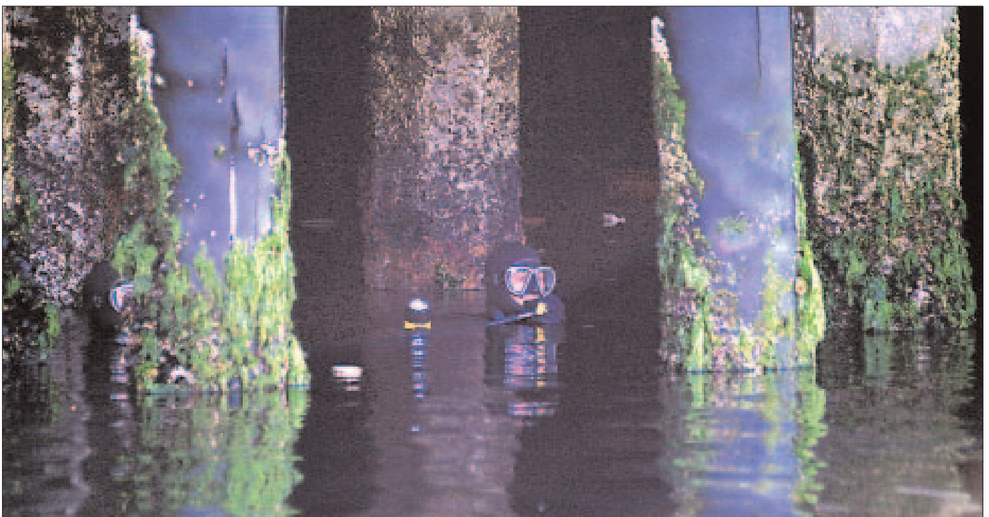
A Coast Guard diver inspects a portion of the 1,650-foot pier that needed to be cleared for the arrival of a Navy ship.
